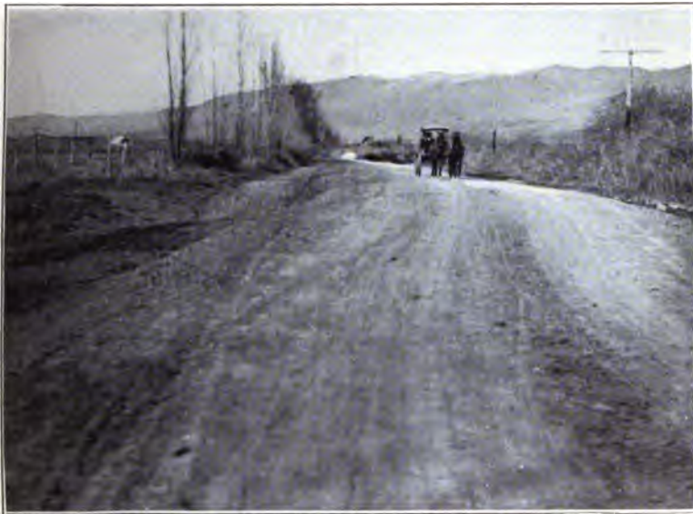
FIG. 14. ROAD NOT STRAIGHT, GRADE NOT UNIFORM, AND CROSS SECTION OF DRAIN DITCHES NOT CONSTANT. ALL THESE CONDITIONS COULD HAVE BEEN GREATLY IMPROVED WITH VERY LITTLE ADDITIONAL COST
